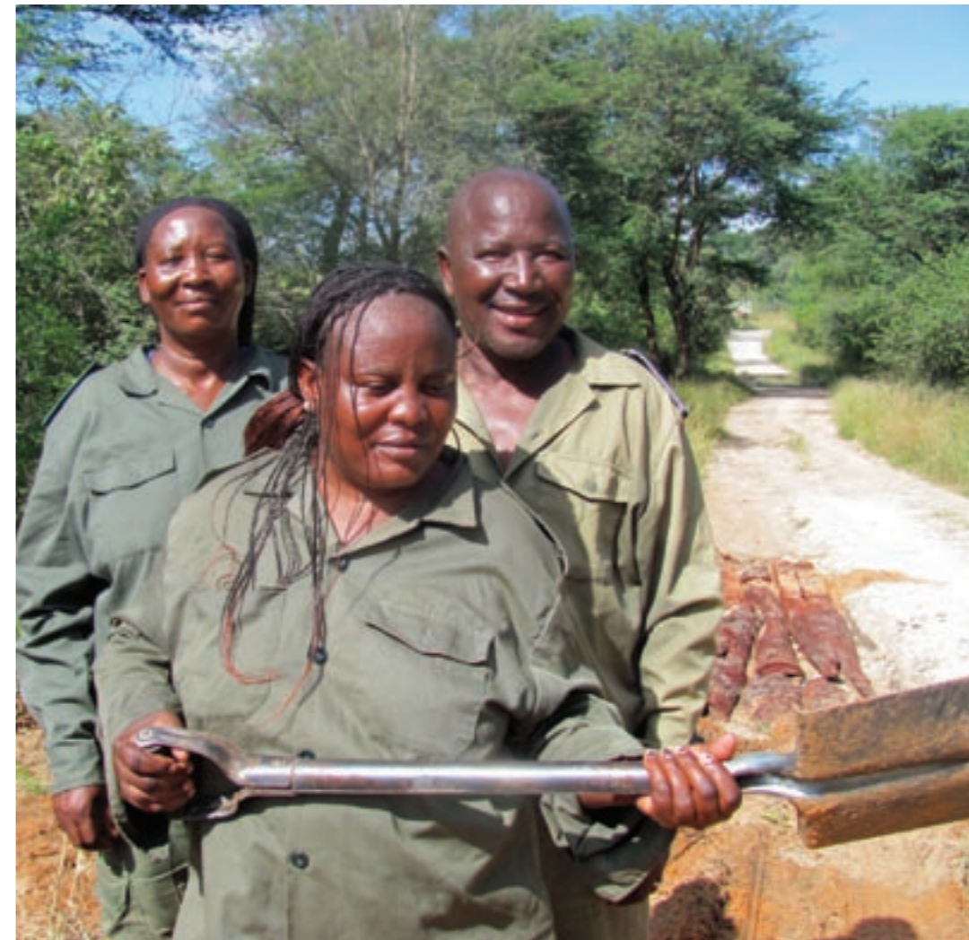
MET staff are the custodians of Namibia's PAs on behalf of the citizens of the country. Here Bwabwata National Park staff are repairing the tourist road to Susuwe Station.
